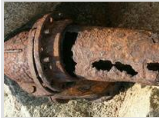
Photo 5: Erosion corrosion and channel rot
