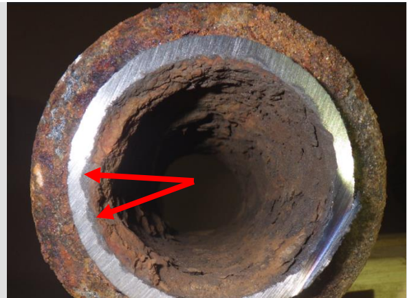
Photo 2: Arrows point to graphitic corrosion that penetrated the pipe wall
