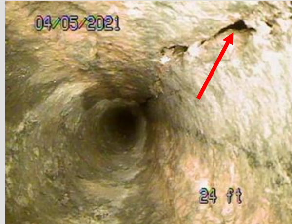
Photo 6: Stress crack corrosion
