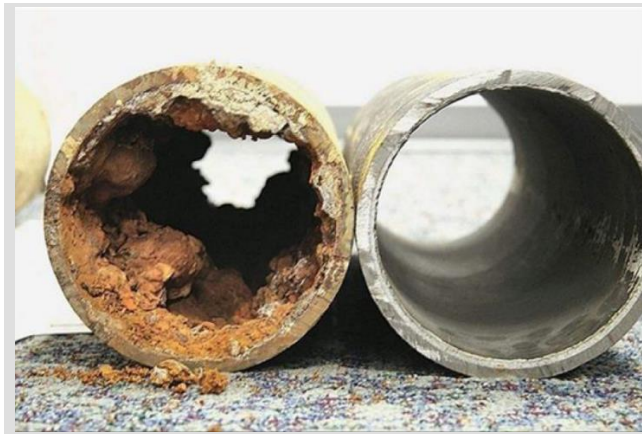
Photo 1: An example of graphitic corrosion with distinctive tubercle formation
